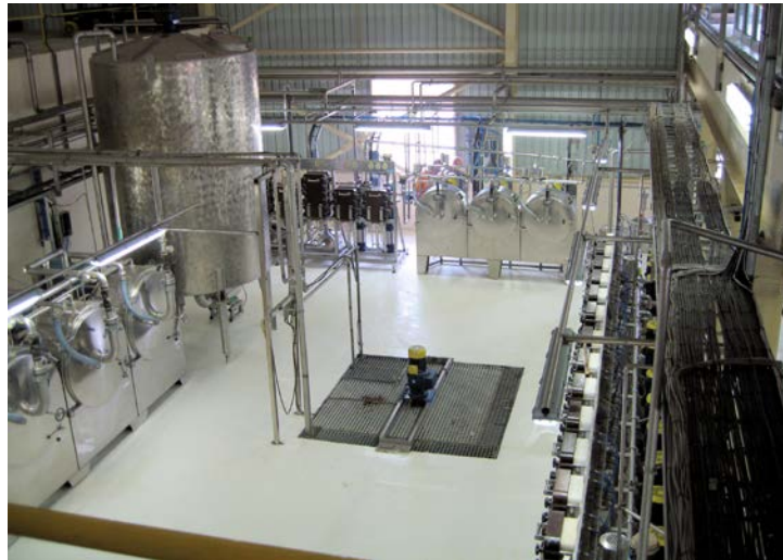
Factory Hall for a capacity of 4 t/h of cassava starch.
